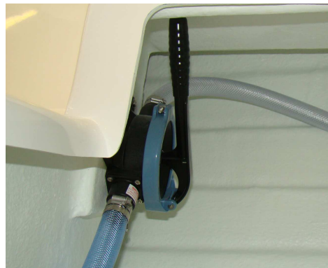
Hand bilge pump inside engine compartment
